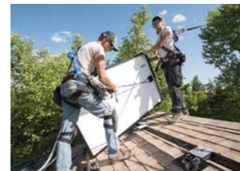
SolarEdge at home
